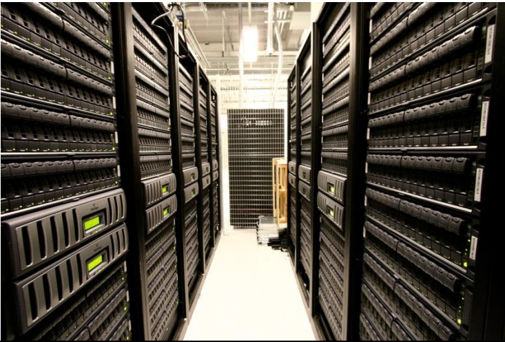
Inside view of a data center.
