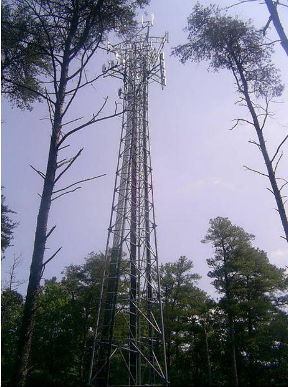
This cell tower is part of a wireless access network.
